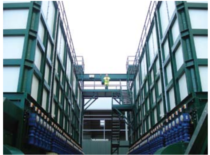
The VCU™ system at Keenan Recycling, Aberdeen, Scotland
